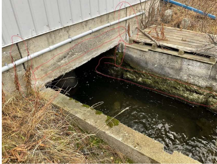
Figure 26: degraded concrete on tailrace walls
