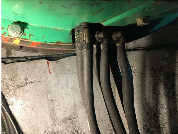
Figure 20: MV Cables Under Generator
