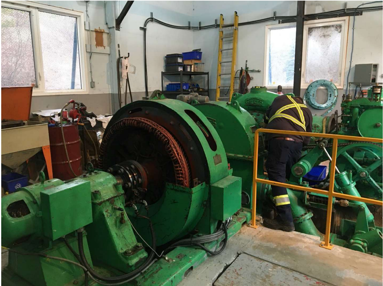
Figure 1: Turbine and Generator
