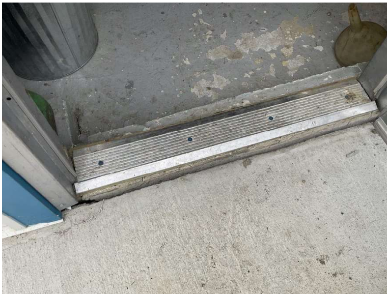
Figure 27: Differential settlement outside and inside the building
