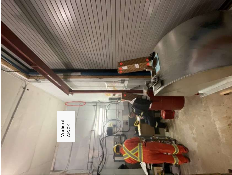
Figure 28: Cracks on main columns
