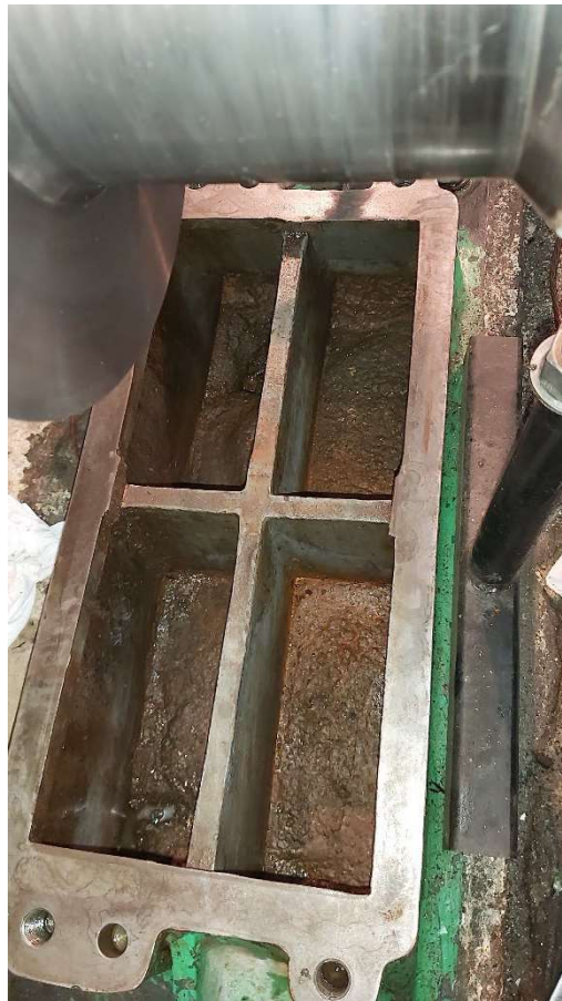
Figure 8: Turbine Bearing Pedestal Hole to Ground
