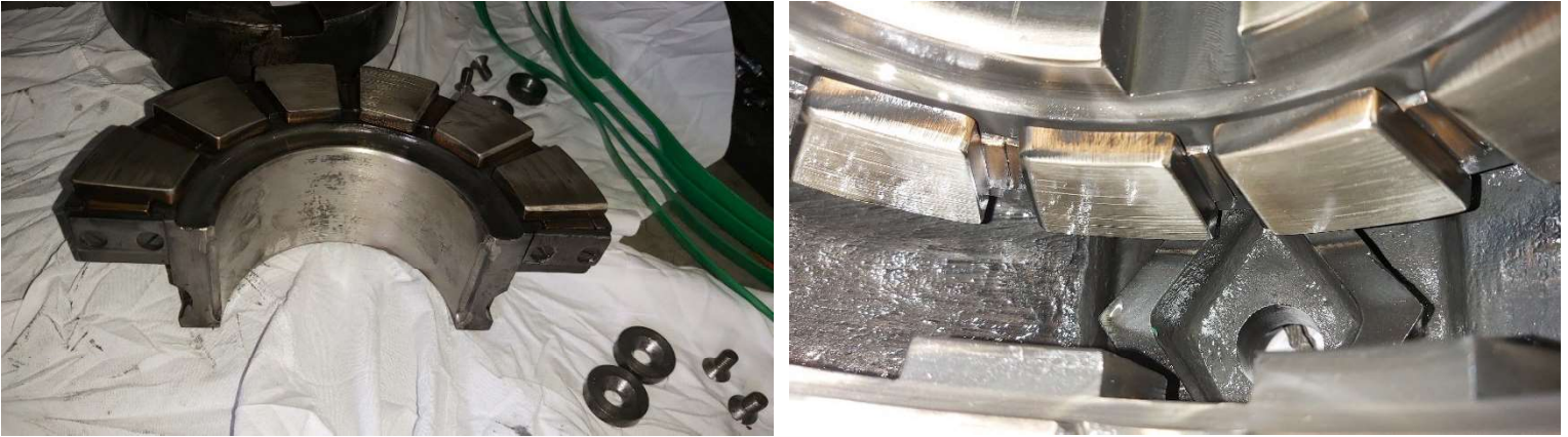
Figure 7: Thrust Pad Damage
