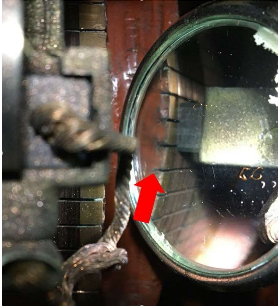
Figure 18: Commutator Remaining Surface (~3 to 4mm)
