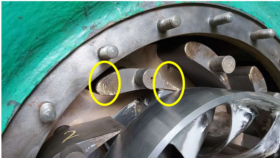
Figure 4: Wicket Gate Damage
